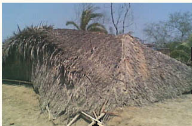
The cyclone-damaged school
